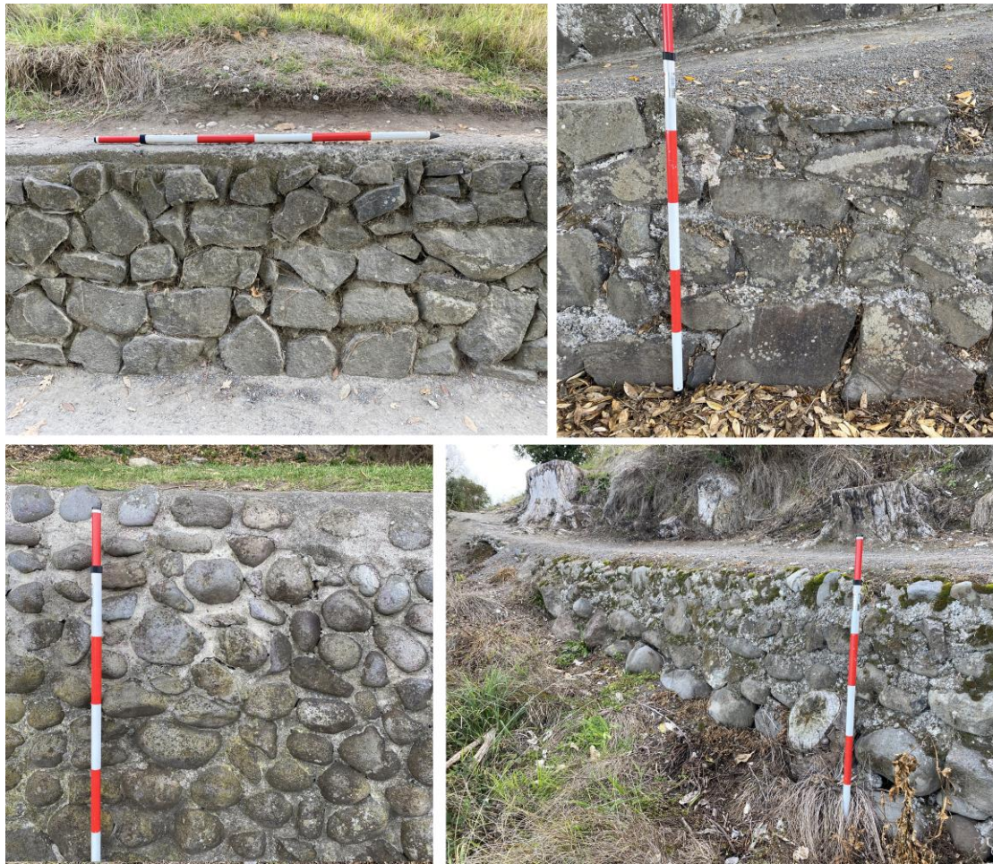
Figure 4 – Comparison of wall masonry styles. Clockwise from top left: Wall 1, Wall 5, Wall 8 and Wall 11.
